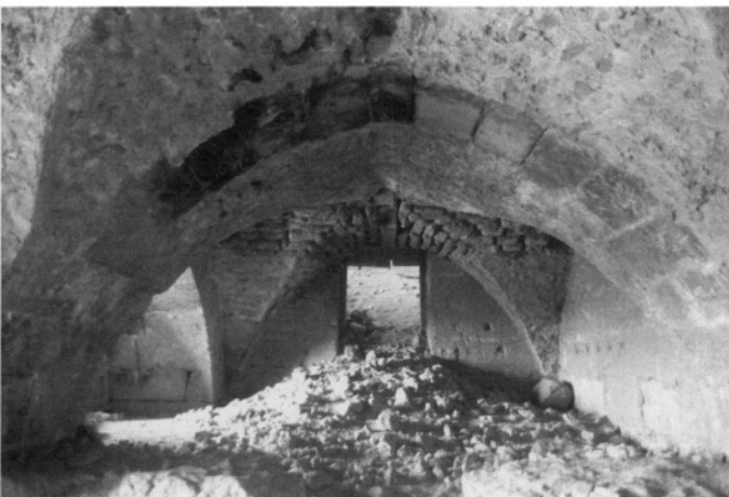
23. Groin vault in the lower hall under the site of the Qaşr al-Ablaq
