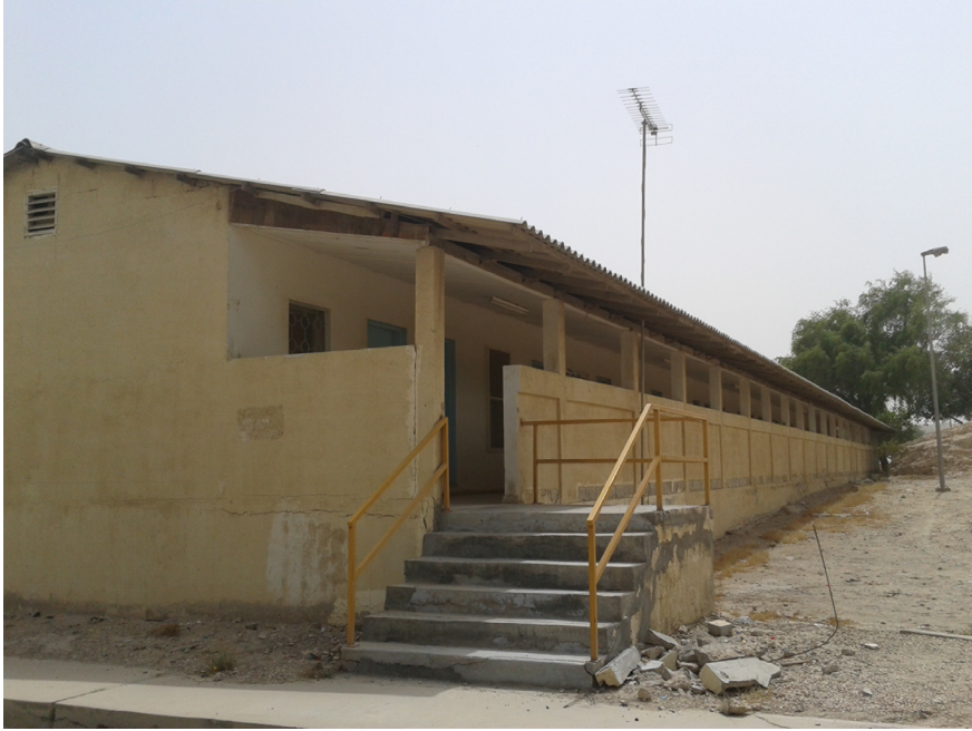
FIGURE 9 Old oil workers' dormitories (former general camp) on the campus of the King Fahd University of Petroleum and Minerals in Dhahran in 2013, Claudia Ghrawi
