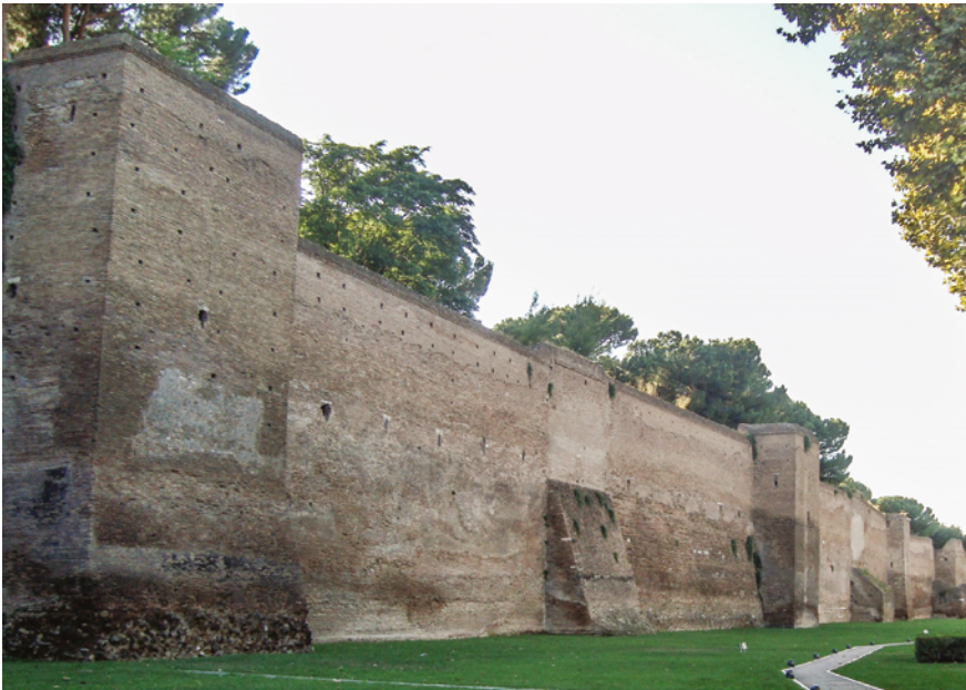
FIGURE 7.2 Rome, section of the Aurelian wall near Porta Metronia PHOTO: LPLT / WIKIMEDIA COMMONS
