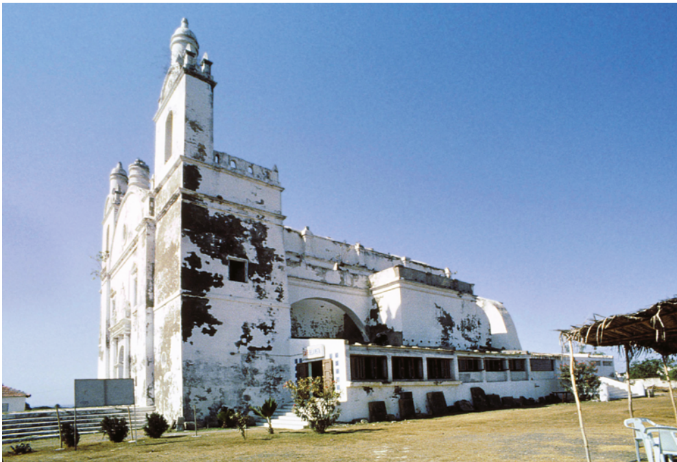
PLATE 4.48 St Thomas's Church, north façade from the northern churchyard. The additional chamber can be seen in the middle of the original wall with a retaining vault between the chamber and the north tower and a flying buttress to the right of the chamber. The extension to the right is a later addition and the colonnade with a light roof in front is modern. In the churchyard numerous inscriptions are kept, some of them leaning against the wall of the colonnade.
