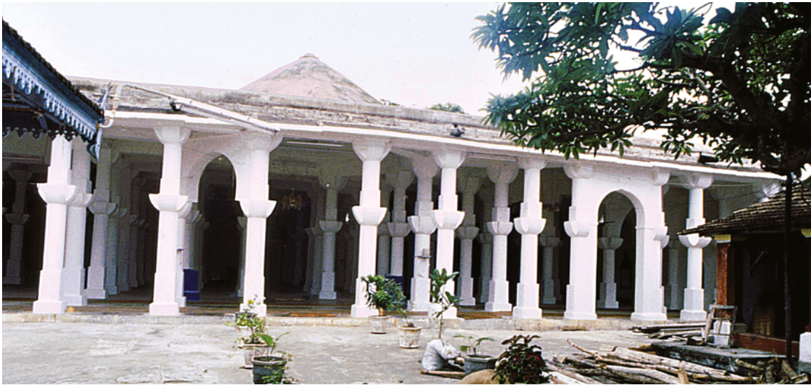
PLATE 4.20 Karao Jāmi', exterior of prayer hall showing later added arches where the stone lintels supporting the roof have cracked.
