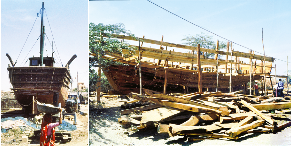
PLATE 6.33 Vanakbara, ship-building yards to the south of the town on or near the demolished site of the Forte de Barra . Left: a ship being refitted; right: a new ship being built with imported wood.
