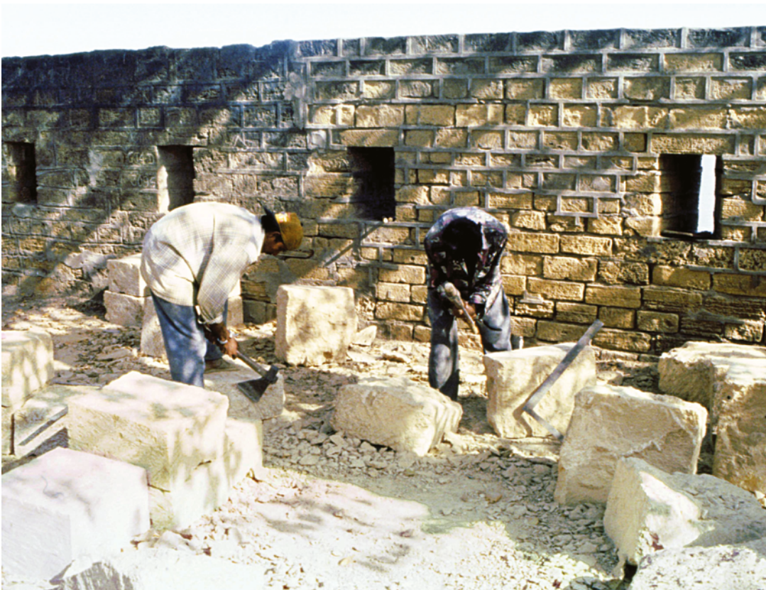
PLATE 3.3 Stonemasons using masonry axes to dress the soft local stone, for use in the restoration of the fort, such as the new wall behind them.
