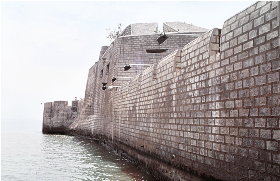
PLATE 3.46 Forte do Mar, northern wall seen from the platform of the northern entrance looking east. The bulging lower part of the middle tower serves to reinforce the massive walls above it. The two openings on the wall of the keep are apertures for cannon, but also provide light for the otherwise dark chambers housing the cannons.
