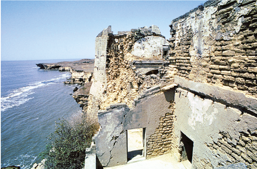
PLATE 3.40 The site of the vestry of St James's chapel, apparently demolished in the 1961 mortar attack. The room with the traces of a sloping roof in the foreground is an antechamber with a door at the right opening to the choir and another door to a larger chamber which must have been the vestry. Behind the fallen wall the eastern end of the nave can be seen, with a window to the roof of the trapezoid area which adjoins the chapel and the fortifications, and St James's Tower visible behind the nave.
