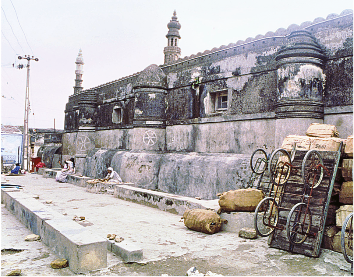
PLATE 4.11 Karao Jāmi', western ( qibla ) wall, exterior. The projection of the three mihrābs is characteristic of the thirteenth and fourteenth-century mosques of the Sultanate of Delhi, but the practice continued in later dates. The floor of the mosque is at the level of the first step of the projection of the mihrābs . The platform and the steps, where some people are sitting, are modern, yet the street level seen at the left corner is still higher than what it was in the early fourteenth century. Building a mosque on a high platform, to give a lofty appearance, was a common practice during the Delhi Sultanate.
