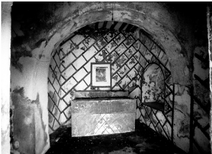
PLATE 3.50 The Chapel of Our Lady of Victories, interior. The light ceiling built with wooden rafters shows that it was not built into the solid south-east banquette, but is a later addition with a lighter structure.
