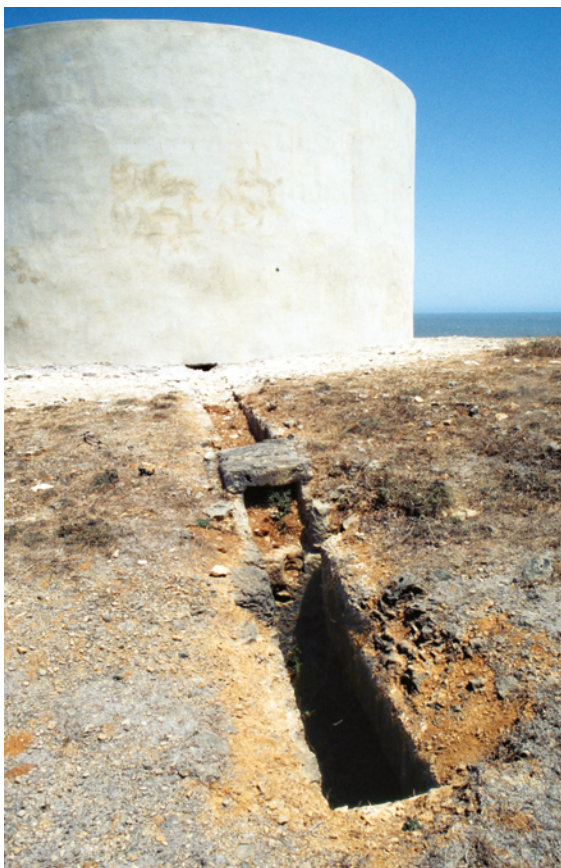
PLATE 5.16 South Tower, view from the western side of the dakhma showing the drainage ditch which has lost its covering slabs leading to the pit, still covered, the edge of which can be seen in the foreground.
