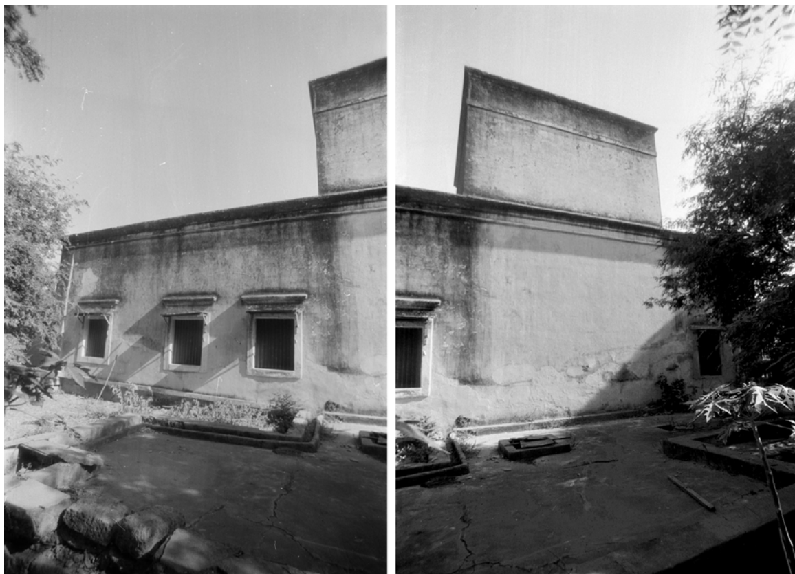
PLATE 5.7 Fire temple, left: eastern side of the southern wall of the fire temple showing the plinth and the cornice of the building as well as the windows of the rooms (f) and (g). Right: eastern side of the wall showing the blank wall of the southern domed chamber (i) and the chamber which conceals the dome at roof level. The window to the right opens to a room (j).
