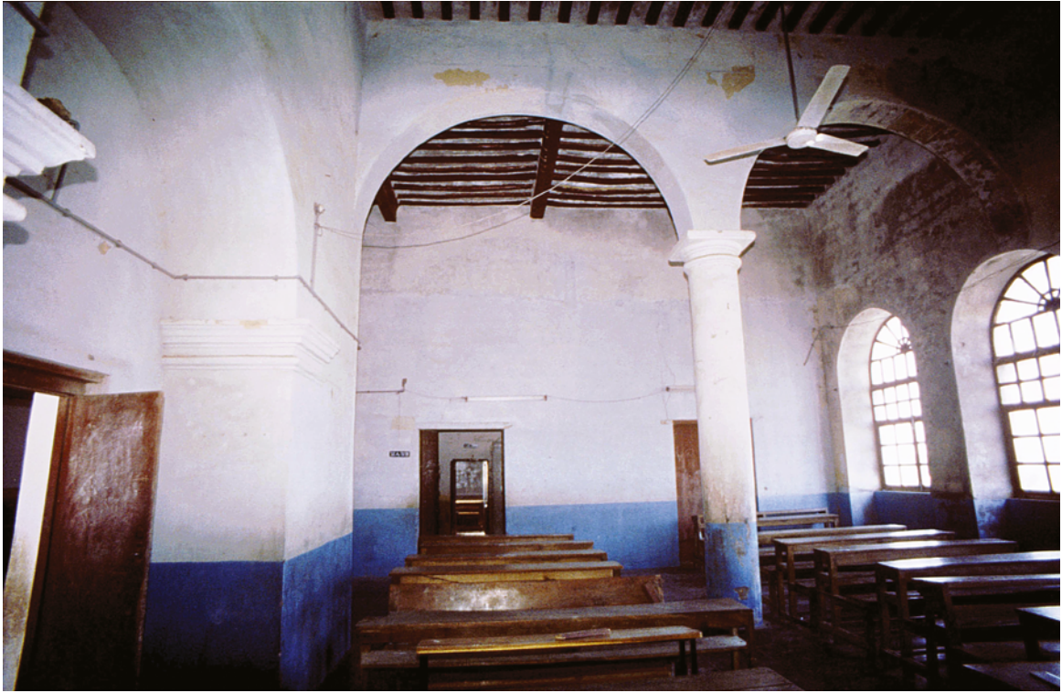
PLATE 4.61 St Paul's Seminary, upper room at the far end of the eastern side with a light roof supported by wooden beams and rafters. The arched windows to the right are part of the row of windows seen on the eastern elevation.
