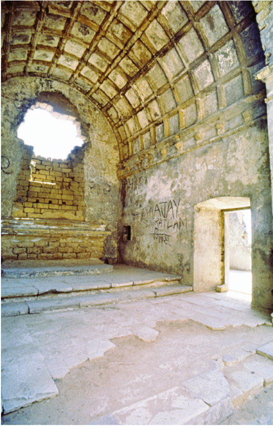
PLATE 3.39 St James's chapel, the choir from the north-west looking towards the door to the ante-chamber of the vestry and the altar, constructed with stone and plastered over. The niche in the eastern wall was partly damaged, apparently by a mortar shell in the Indian Navy attack of 1961, but has been repaired later. The barrel vault, however, is intact and is decorated with plaster coffering in the style of a wooden ceiling.
