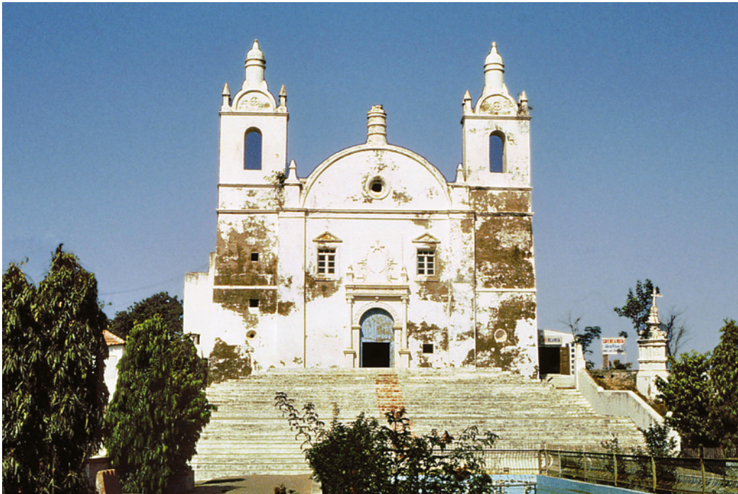
PLATE 4.43 St Thomas's church, eastern façade with a semi-circular gable reflecting the profile of the vault of the nave and flanked by two belfries, which no longer retain their bells. The shaft above the gable bore a cross originally, shown in our drawing of the façade. The wide flight of steps ascending to the terrace in front of the entrance can also be seen, and the cruzeiro to the far right.
