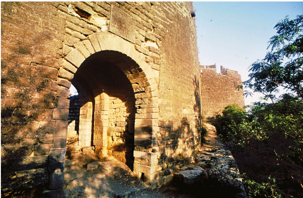
PLATE 4.29 Western town wall, southern postern gate (m in map) from north-west. The stonework of the gate is not properly keyed to the wall showing that the gate might have been opened some time after the construction of the wall. Above the gate is the in situ inscription of Aires Telez, the captain of Diu in the 1570s, who was also responsible for the construction of the wall and the northern postern gate. The platform in front of the gate lead originally to a drawbridge, no longer extant.
