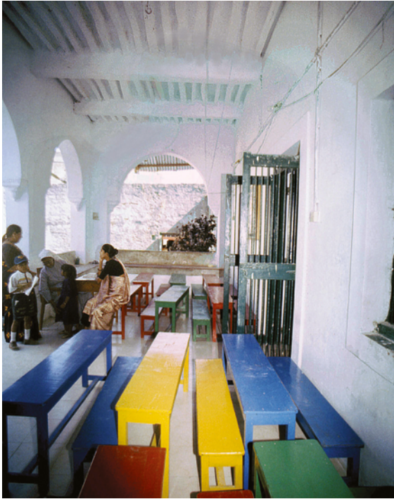
PLATE 5.2 Former fire temple, now St Anne's Convent School, western portico (a) looking north with the door to a hall (b) at the right. The exposed wooden structure of the ceiling can also be seen.
