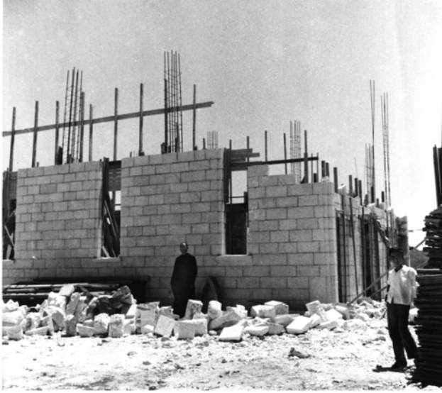
FIGURE 3.1 Construction work on the new church and vicariate in Amman, 1950s APLJ/AEBAF
