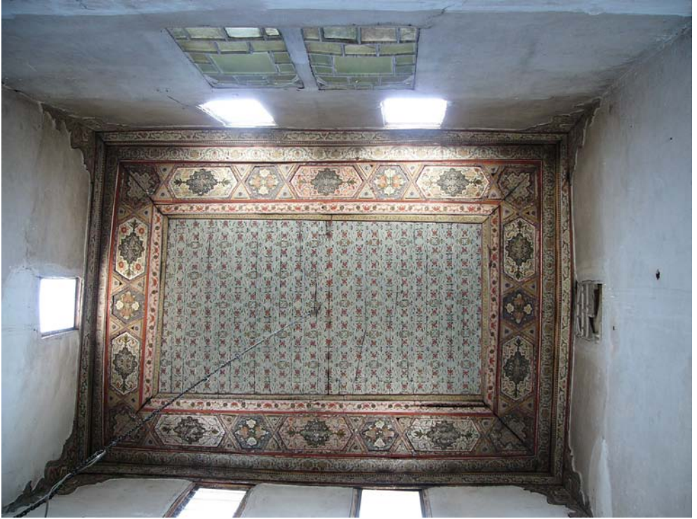
FIGURE 17.26 Bayt al-Qaziḥa, qā'ā in the west wing of the house, ceiling of the ground-level entry space ( ataba ), which is preserved with its original light, fresh colour scheme
