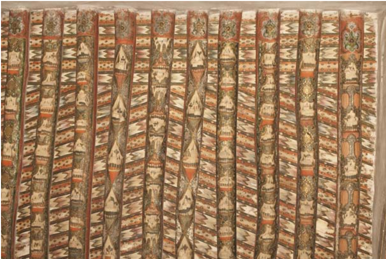
FIGURE 17.20 Bayt Sa'īd al-Quwatli/al-Murādi, inner courtyard ( ḡuwwāni ), detail of a šīša ceiling in the north wing PHOTO: MECHTHILD BAUMEISTER, 2008
