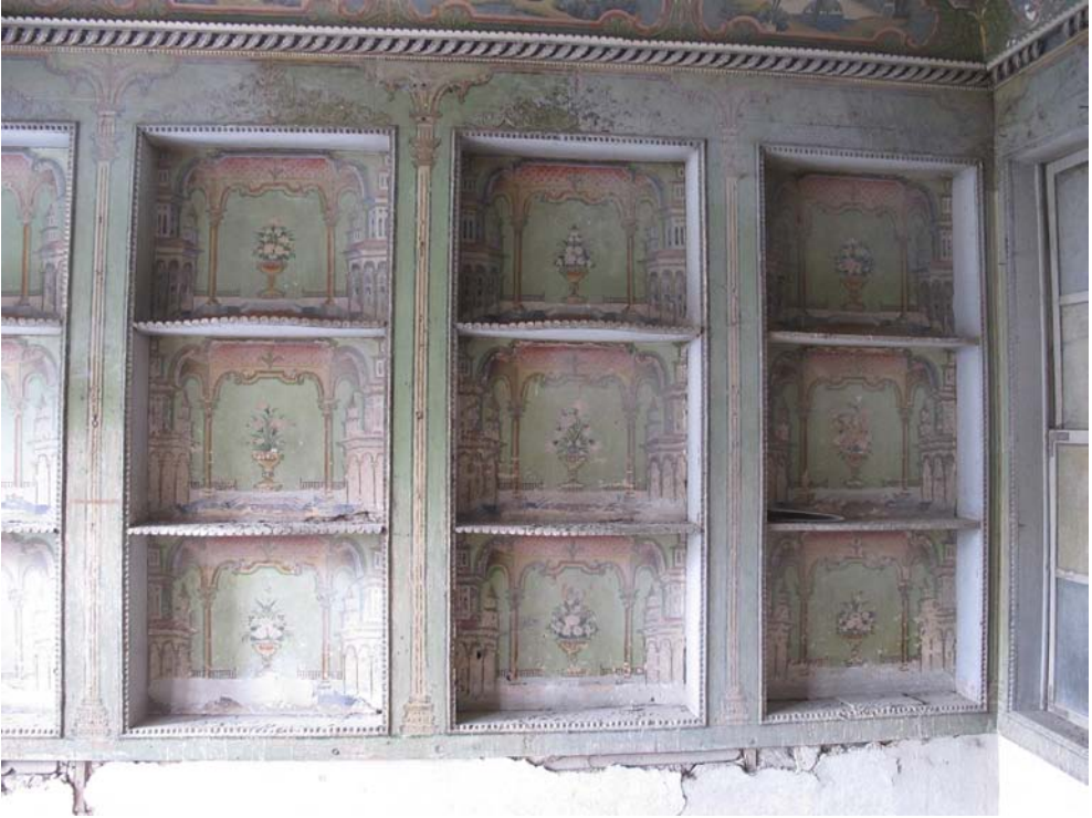
FIGURE 17.32 Bayt ‘Abd al-Qādir al-Ġazā’irī, house in the middle of ‘Abd al-Qādir’s five adjacent houses, room on the first floor of the south wing, west wall with characteristic mid-nineteenth-century niche decoration PHOTO: ANKE SCHARRAHS, 2011
