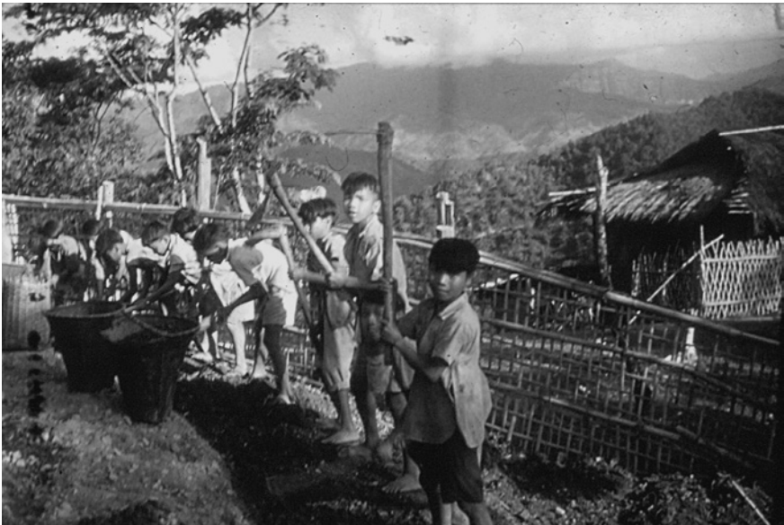
FIGURE 9.6 Communal labor. Boys repairing a road in Sihfa village, c. 1956. PHOTOGRAPHER UNKNOWN (POSSIBLY GWEN REES ROBERTS). REPRODUCED BY PERMISSION OF AIZAWL THEOLOGICAL COLLEGE COLLECTION, AIZAWL, MIZORAM, INDIA
