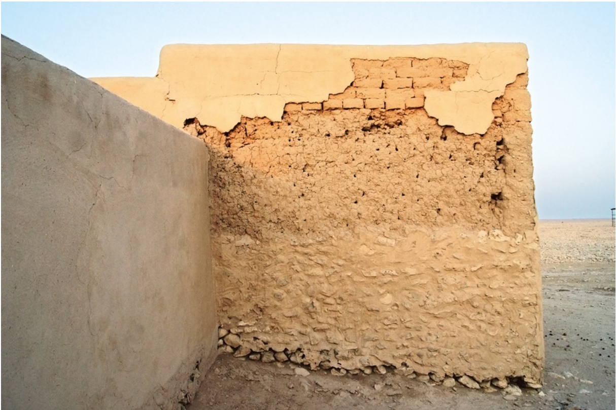
FIGURE 8.20 Qal'at Rakayat: close up of wall face with stone base, historic mud bricks and restoration mud bricks (from 1988). PHOTO: M. KINZEL, QIAH/UNIVERSITY OF COPENHAGEN.
