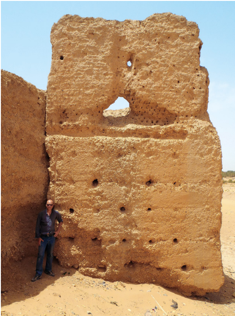
FIGURE 3.9 Tower against the north periphery wall (section 2 in this article). PHOTO: ROMAIN MENSAN 2014.
