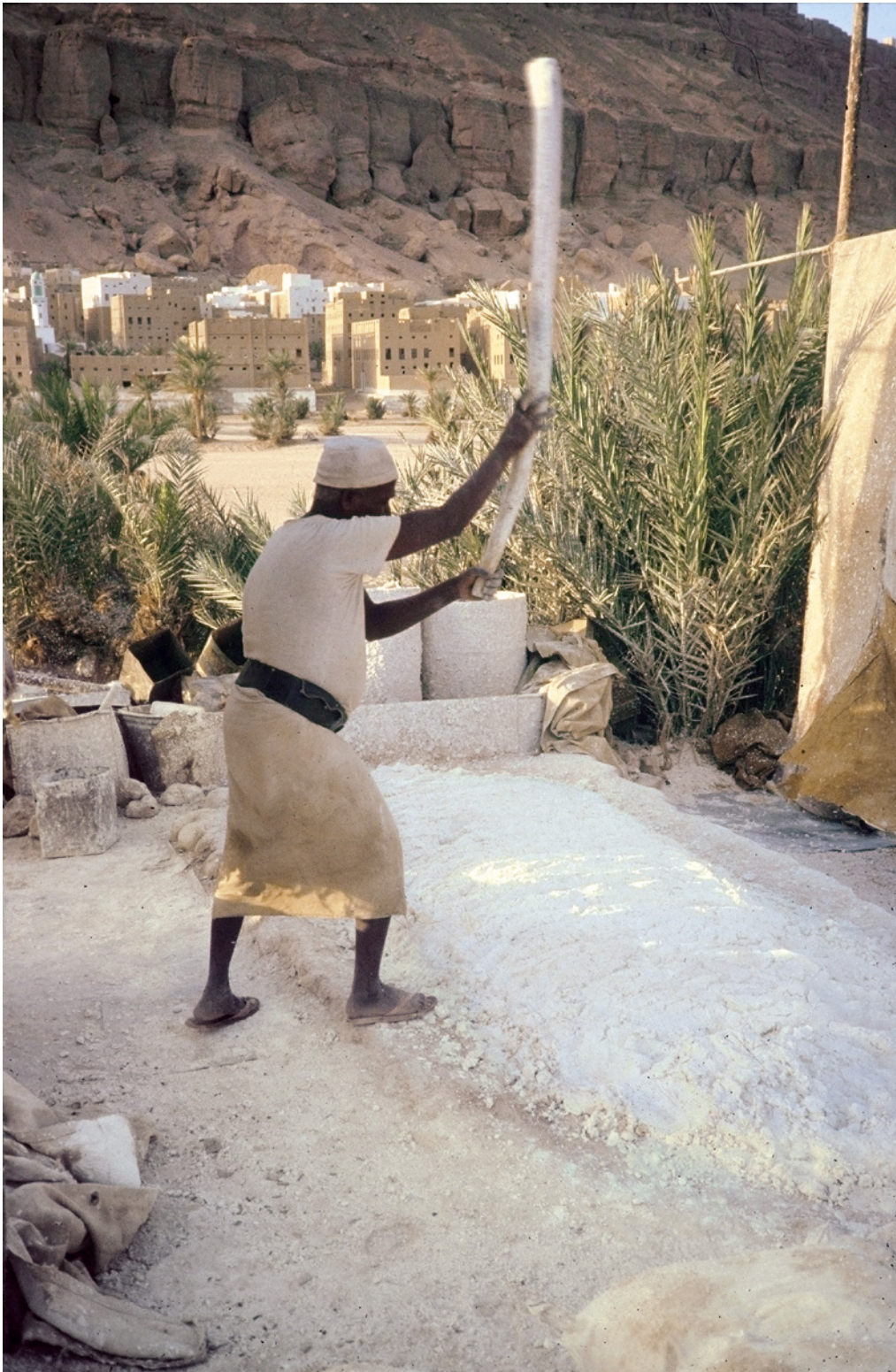
FIGURE 7.18 Lime-based Ramad for waterproofing the upper parts and basements of the houses CREDITS: CHRISTIAN DARLES.
