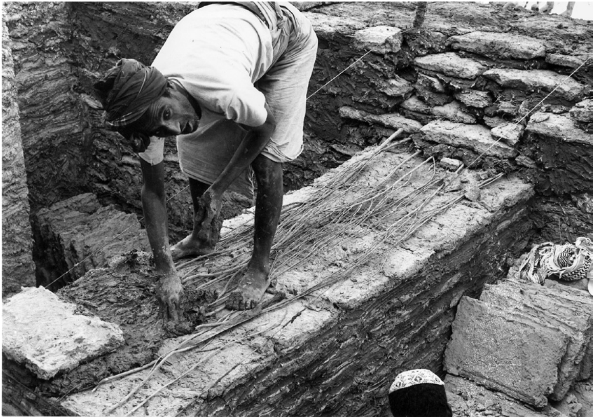
FIGURE 7.19 Branches and timbles enable the clamping of the walls CREDITS: CHRISTIAN DARLES.
