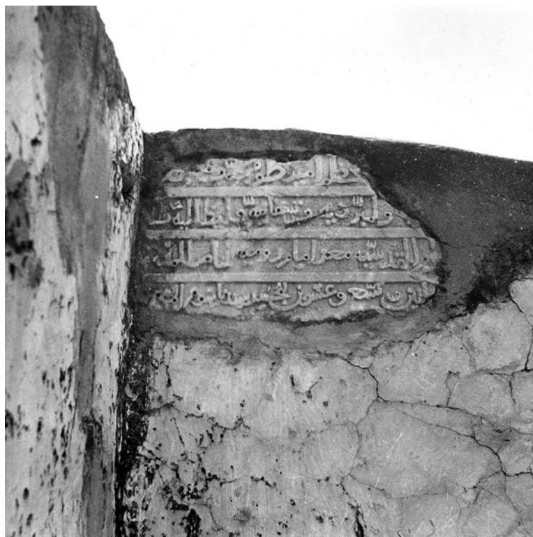
Pl. o8. Inscription inserted into the southern wall of the W. courtyard after repair around 1949. (Photo: Courtesy IAA)
