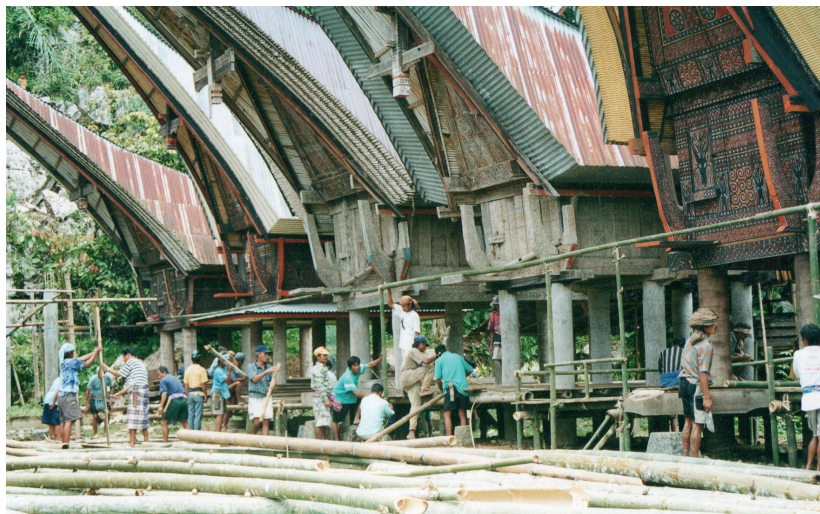
Ill. 6.4. Men constructing a ceremonial field in front of rice barns (photo by Wendy de Jong-Jakobs).
