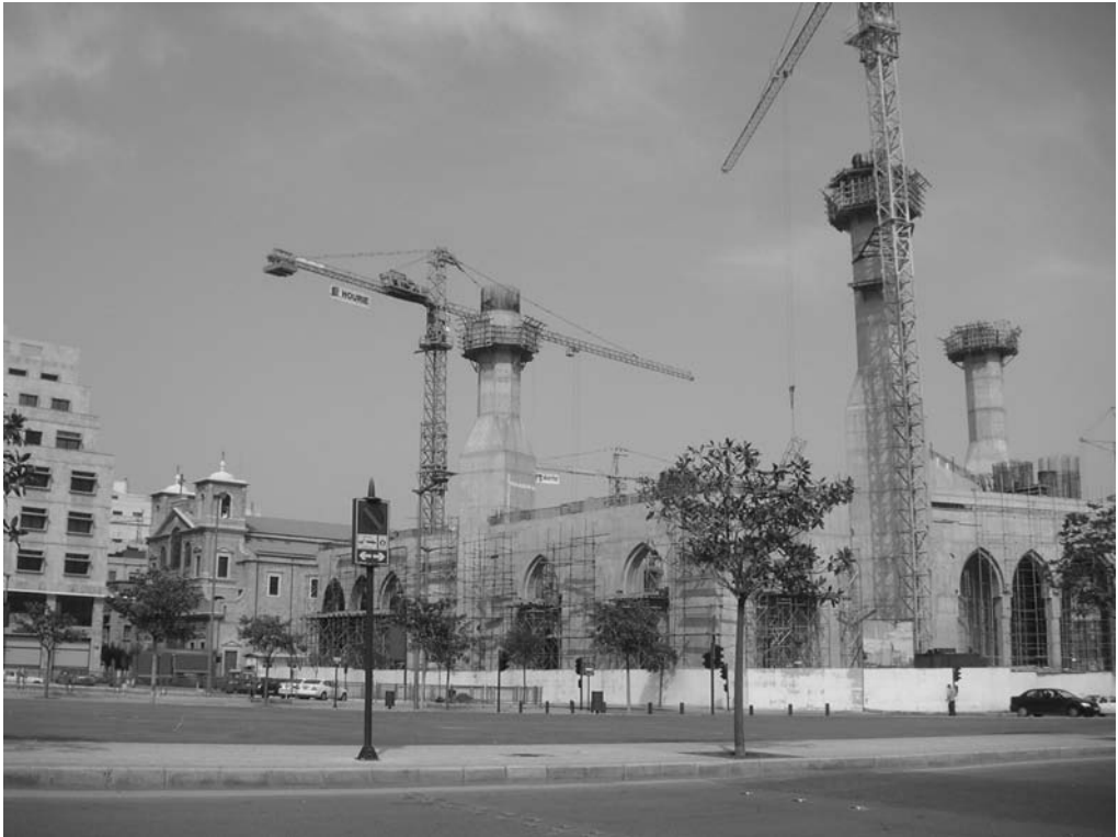
Fig. 10. New mosque under construction (March 2004) between Martyrs Square (al-Burj), in front, and St. George's Cathedral, to the left. At the far left is the Lazarieh complex, developed in the 1950s on property freed up by the move of a religious school. Photo by J. Nasr©.
